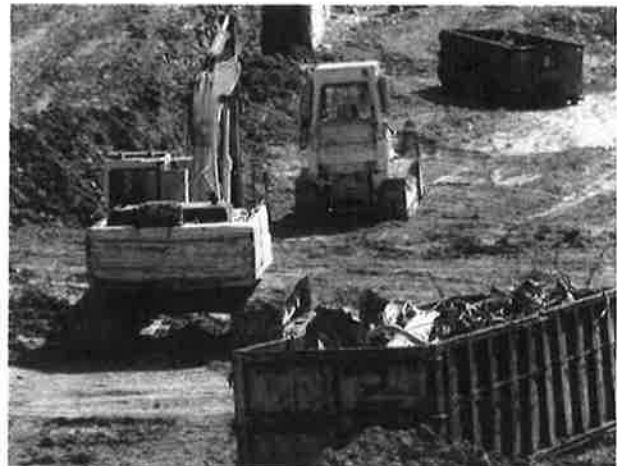
Construction waste should be collected in designated waste collection areas on-site, such as metal dumpsters.
